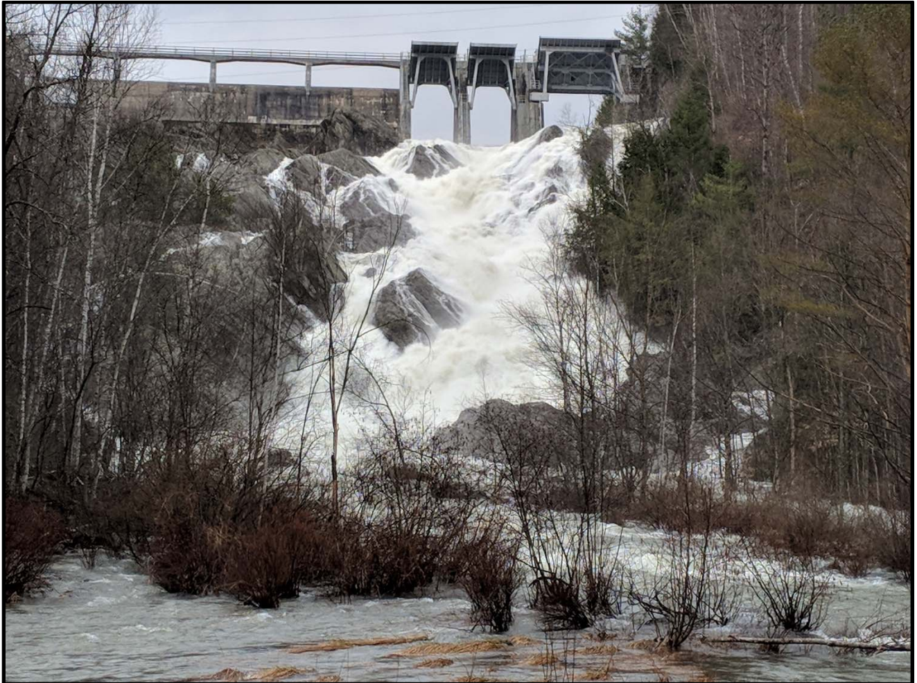
Figure 4: Waterbury Reservoir Dam – Spring 2018 Taintor gates (3) fully open and releasing flow Uncontrolled spillway is left of Taintor gates (releases flow when reservoir levels >617.5 ft)
