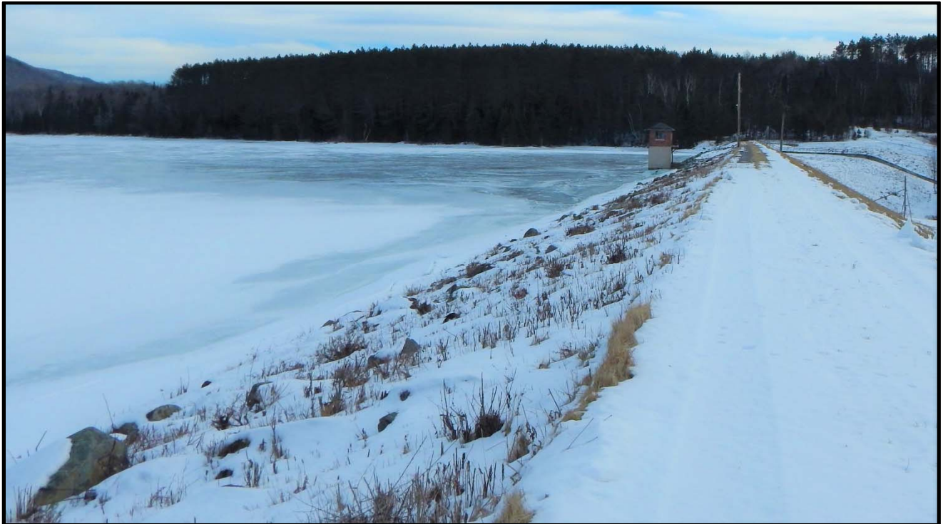
Figure 3: Mollys Falls Reservoir – winter 2015-16, water levels lowered below dam crest providing storage for snowmelt events
